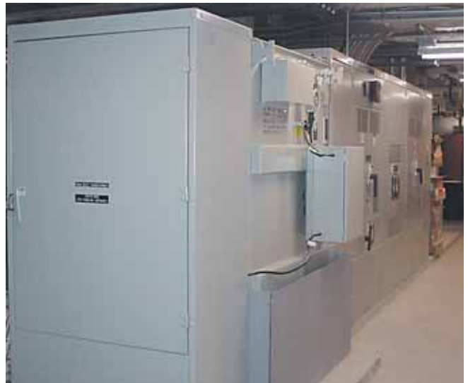
Liquid-filled transformer in Cathedral Place Office Complex, Milwaukee, WI. Containment pan for 100% fluid.
